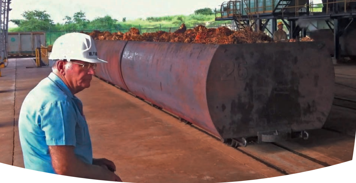
Figure 26: Palm oil extraction plant: Bioplanta Palmera para el Desarrollo S.A., Carepa, Colombia, 2014
